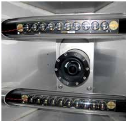
Lights and camera are installed in the photo tunnel
